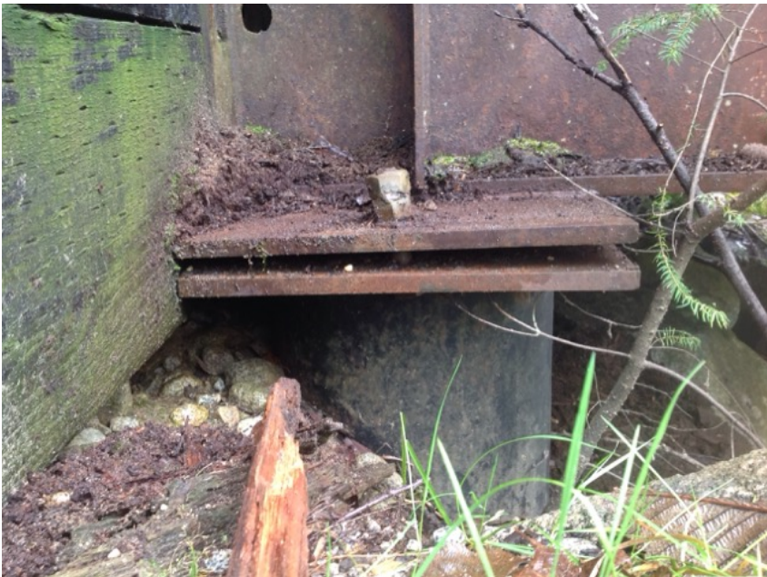
right bank bearing plates offset - holes not slotted and bolts stressed
