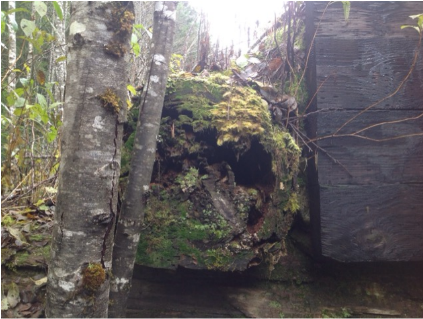
wing logs retaining fill in poor condition
